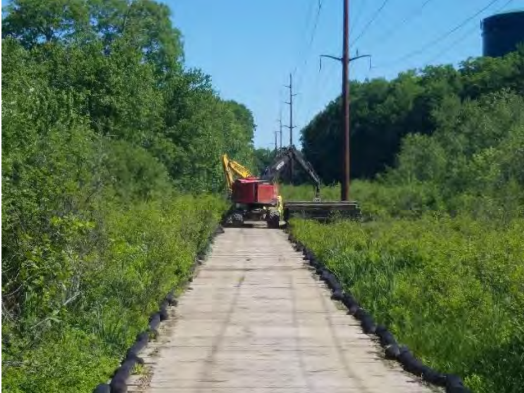
Fig 11: Crew beginning to remove timber mat access road to Str. 35, through wetland DW41. Viewing north. (06-16-20).
