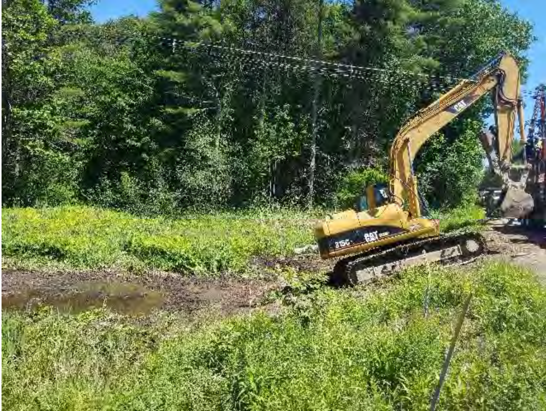
Fig 13: Crew removing timber mat bridge through wetland DW29, off of Route 108. Viewing north. (06-16-20).
