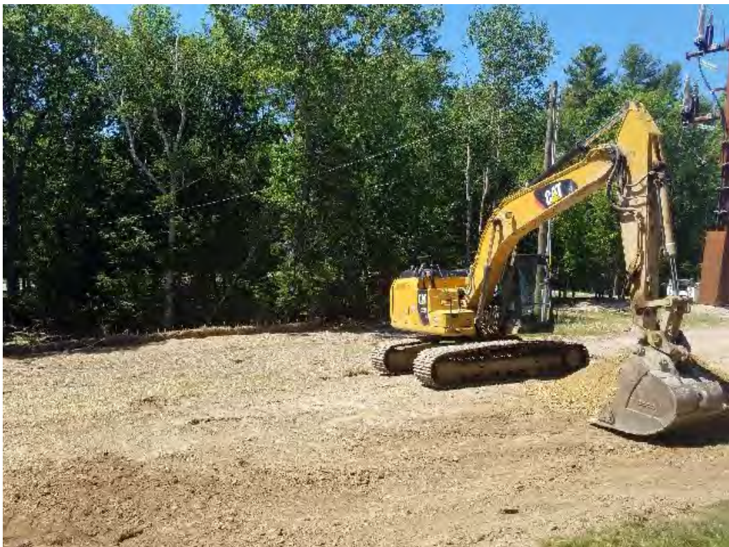
Fig 8: Removing timber mat pull pad at Str. 99 at Getchell property/west side of bay. Viewing south. (06-15-20).
