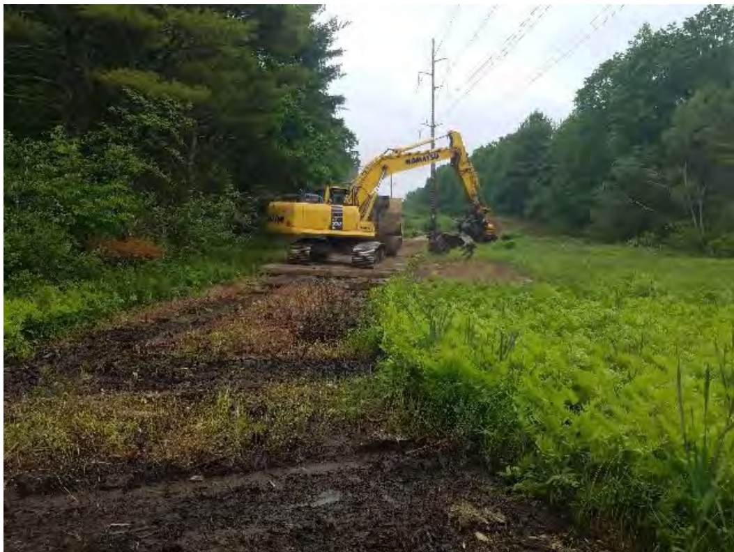
Fig 2: Crew removing timber mat access road between Strs.85-86, through wetland DW24. Viewing southeast. (06-11-20).
