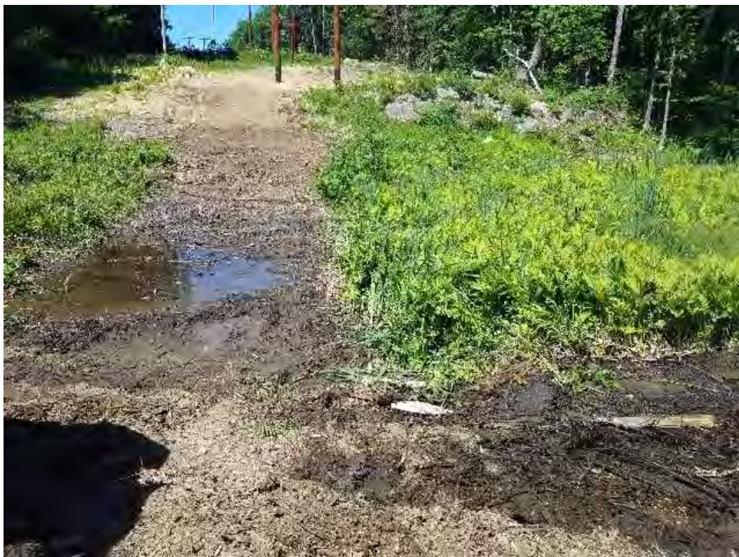
Fig 14: Crew removing timber mat bridge through wetland DW29, off of Route 108. Viewing west. (06-16-20).
