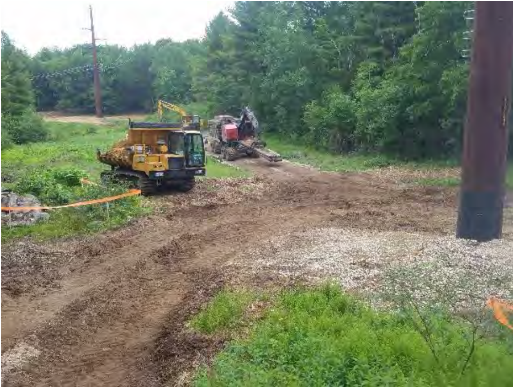
Fig 1: Crew beginning to remove timber mat access road between Strs.85-86, through wetland DW24. Viewing northwest. (06-11-20).
